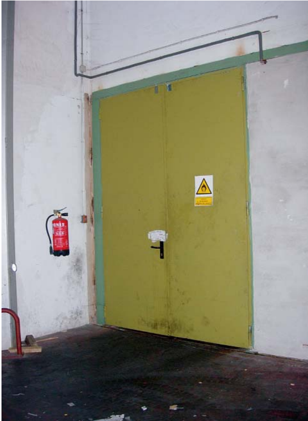
Compartmentalisation with EI doors in flammable-materials stores
