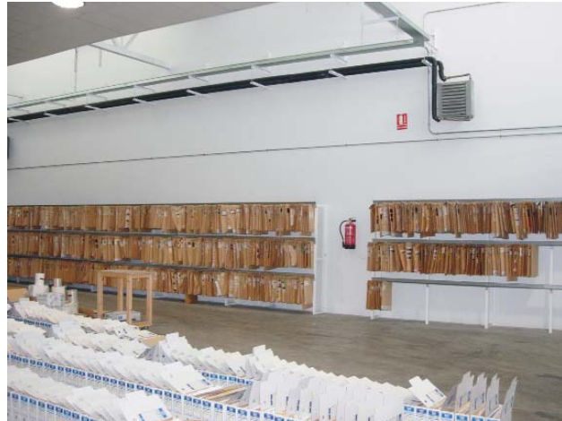
Wall-mounted unit heater
