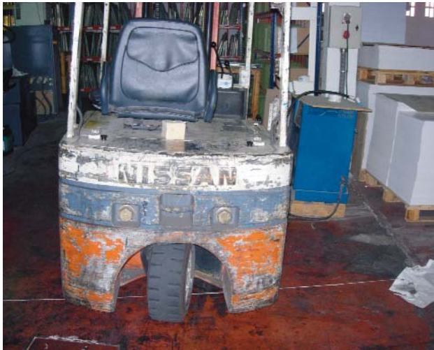
Battery charging with combustible materials (printed paper) nearby
