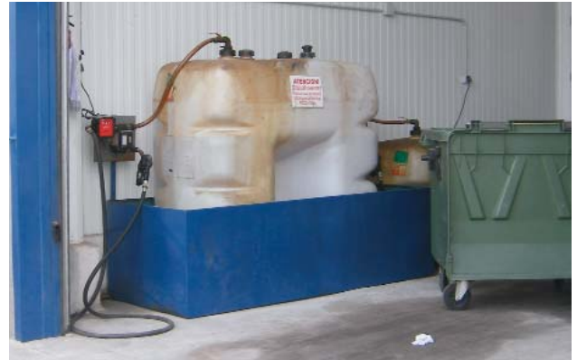
Diesel oil supply tank with spill basin
